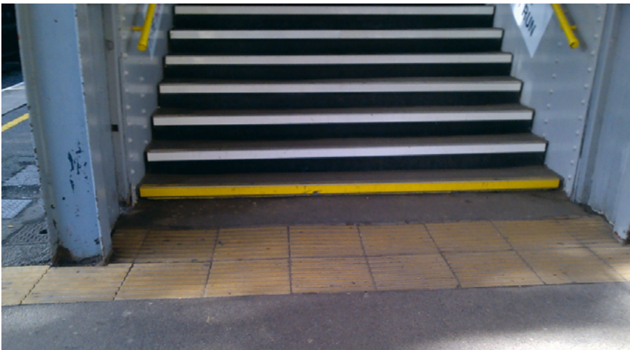
Image 5 - this photo shows ascending stairs with 800mm of buff coloured corduroy paving at the bottom of the last step.
