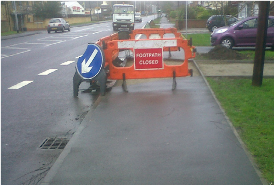
Image 9 - Streetworks can block off pedestrian routes, forcing pedestrians to walk into the road around the barriers.
