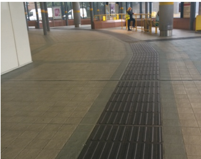
Image 19 – Using tactile guidance paving within stations and interchanges can assist people with sight loss find individual bus bays and other facilities.
