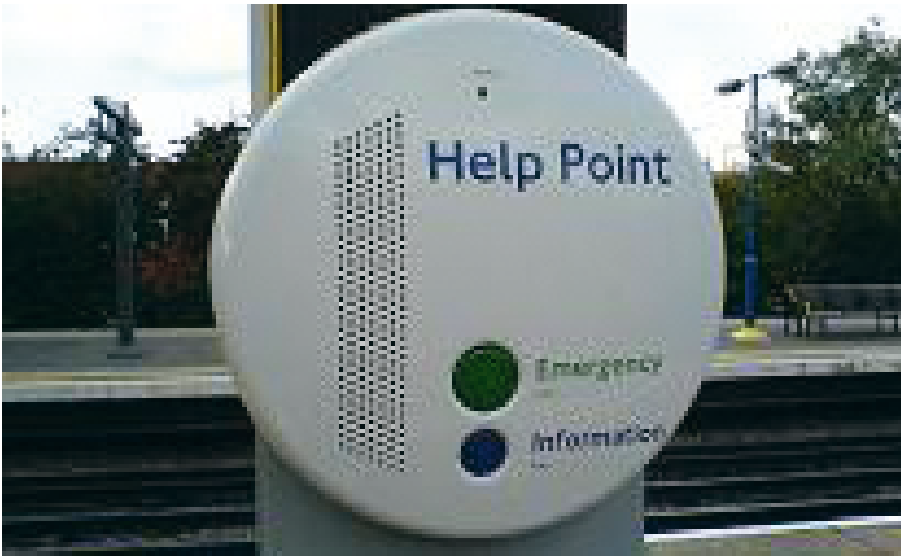
Image 22 - 'Help points' at stations should be easily identifiable, and should have tactile features such as embossed text or braille.
